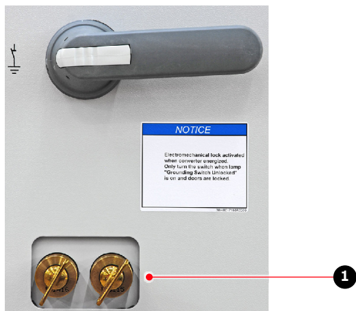
Fig. 17. Example of a customer-specific trapped (1) key interlock system
